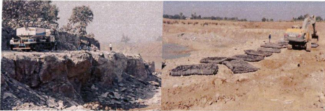
Photograph 2. The charging of the 15 no. RPL bench and use of blasting mate at 7050 RIL blast face to prevent flyrock.
