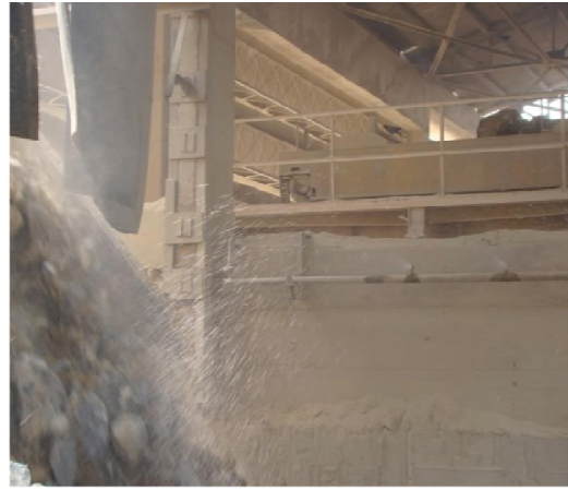
Water spraying System in Crusher Hopper
